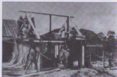
From cutting the timbers in the forest to placing the ridge-beam atop the house frame, indigenous architects combine ritual, design, and construction in a unified building process. House-raising in Madagascar. (Coulaud, The Zufimaniry House: A Witness of the Traditional Houses of the Highlands of Madagascar in Izikowitz, 194.)
